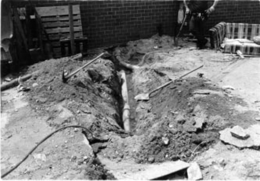
Figure 3 In connection with a regulatory enforcement action, this facility had been forced to cap a pipe that was used to discharge hazardous waste into a leaching pool. When a criminal search warrant was executed years later, investigators saw that the interior discharge pipe was still being used. The parking lot was excavated. Investigators discovered that a new pipe had been added, diverting the hazardous waste to a new, illegal leaching pool
